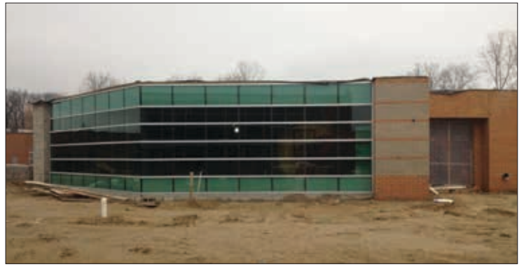
Construction of the new science, art and technology wing is on schedule. This is an exterior view of the new art room.
