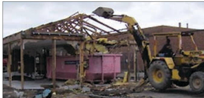
The old weight room is demolished to make room for the new training and fitness building. The new facility will contain space for weightlifting, plyometrics, stretching, rehabilitation and a training room.
